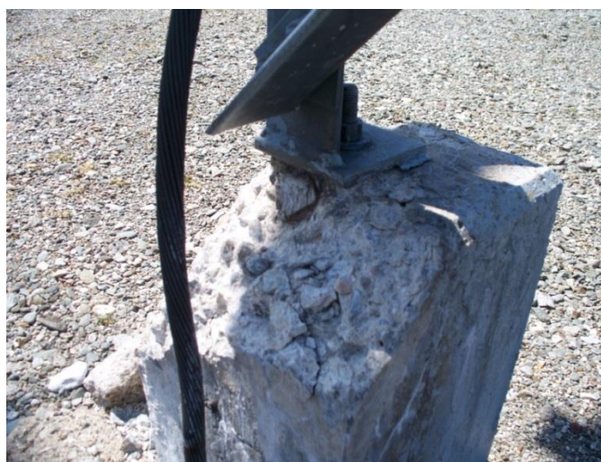
Figure 13: Structure B1T1 Bottom Terminal Stations
