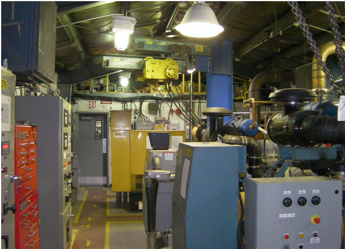
Figure 2: Black Tickle – Diesel Generators in Powerhouse
