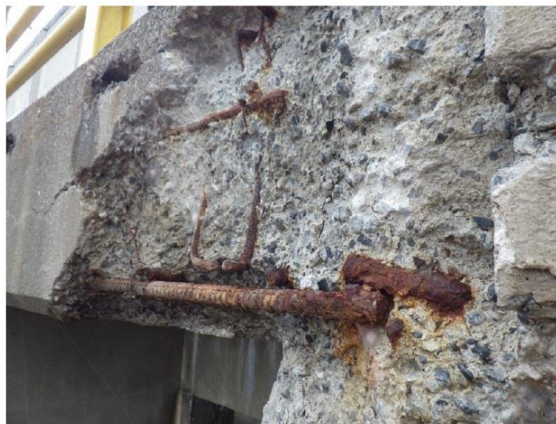
Figure 15: Deterioration on the Draft Tube Deck
