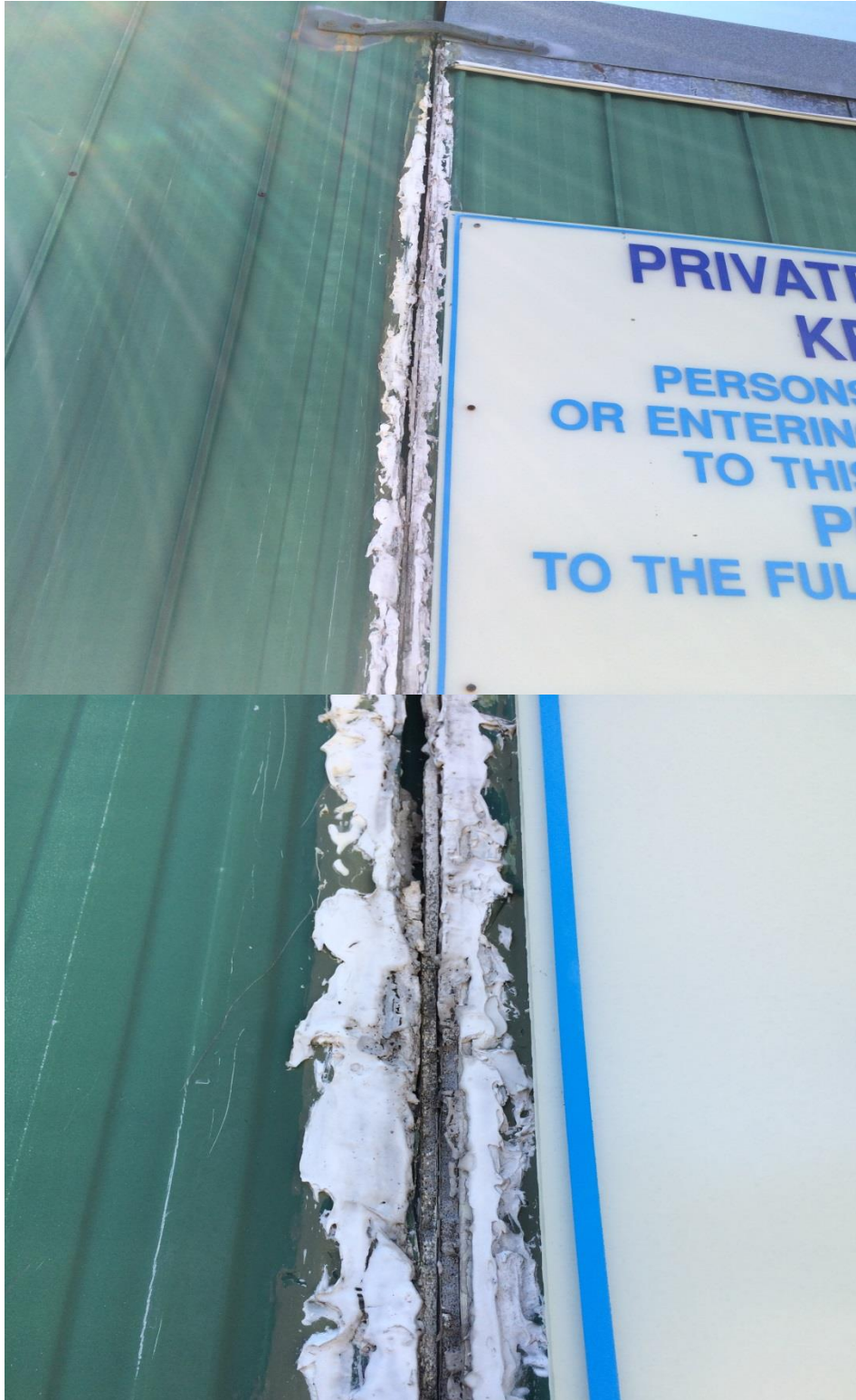
Figure 12A and 12B: Bay d’Espoir Hill – porch separating from main building
