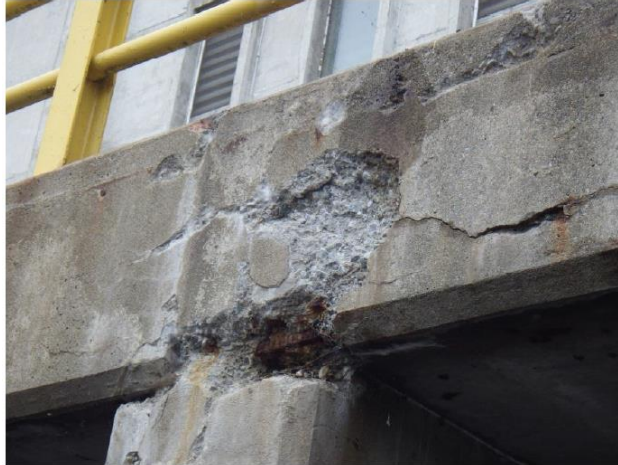
Figure 14: Deterioration on the Draft Tube Deck
