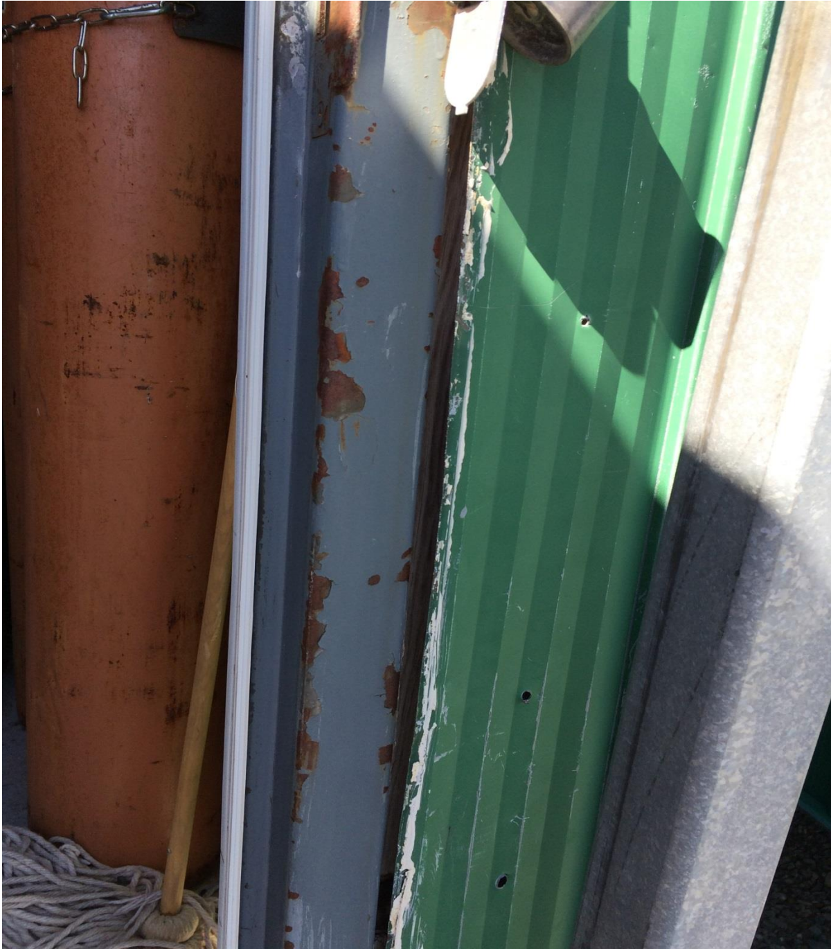
Figure 4: Gull Pond Hill – exterior metal siding – weathered, damaged, and separating from building
