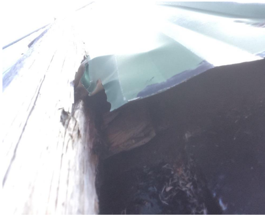
Figure 6: Gull Pond Hill – Damaged siding and exposed sheathing
