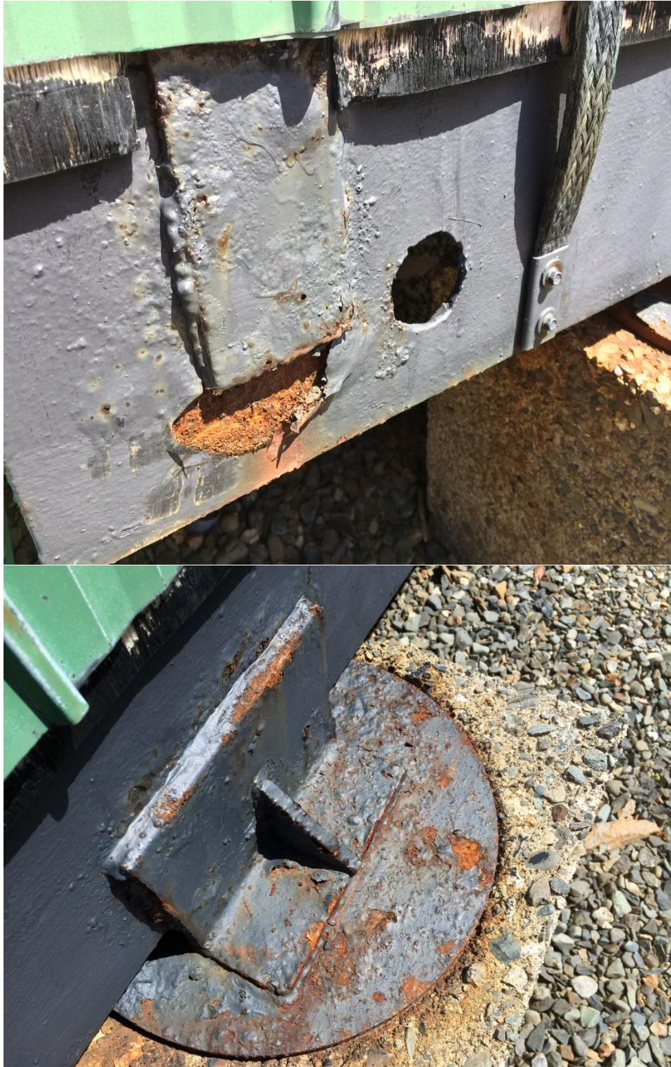
Figure 15A and 15B: Bay d’Espoir Hill – building metal floor frame rusting
