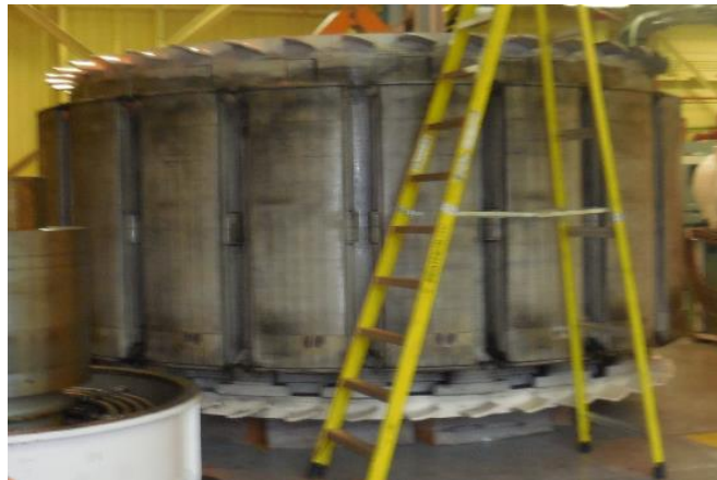
Figure 2: Hinds Lake Rotor – The rotor fans that circulate air to cool the Rotor and Stator are bolted to the top and bottom of the rotor
