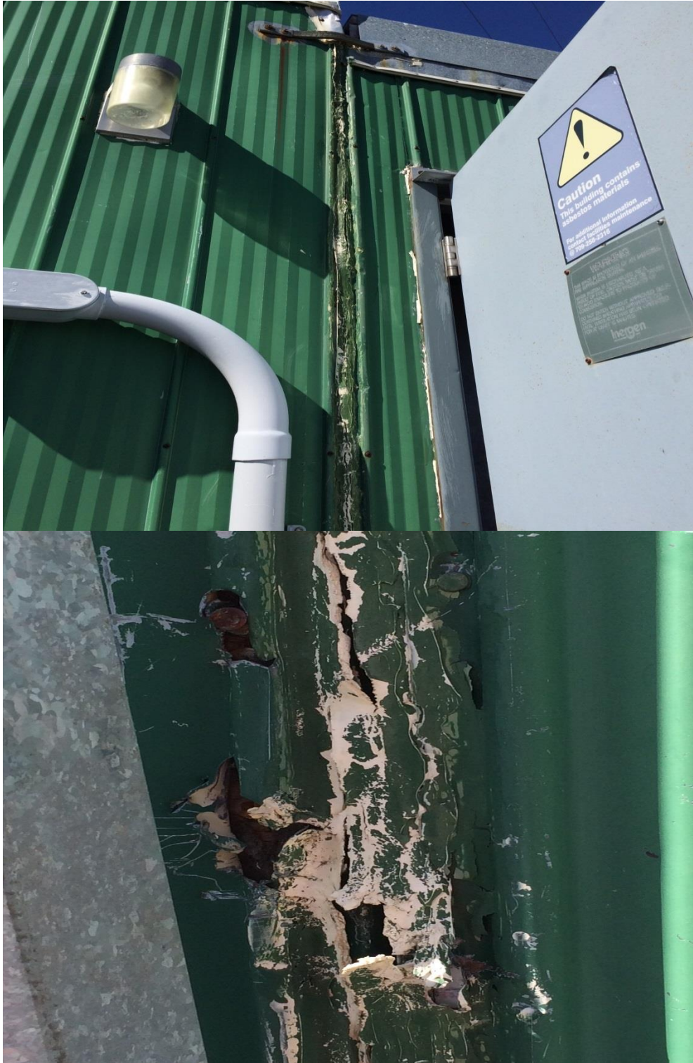
Figure 11A and 11B: Gull Pond Hill – porch separating from main shelter
