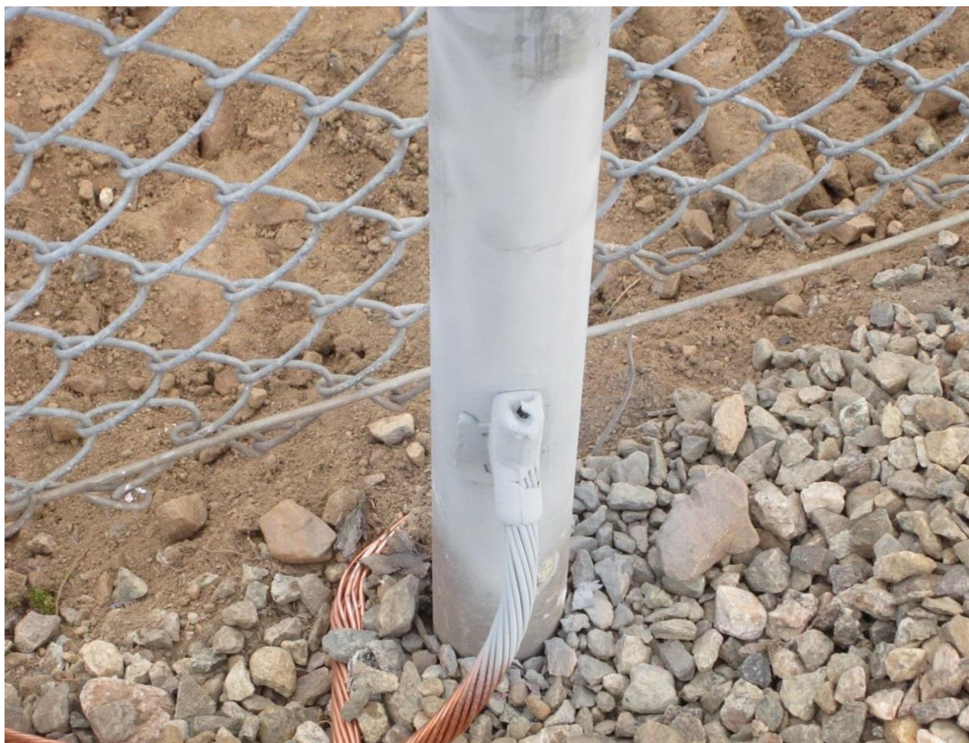
Figure 7: Typical Grounding Connection on Terminal Station Fence
