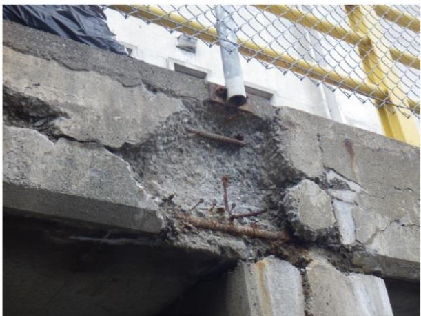
Figure 13: Deterioration on the Draft Tube Deck
