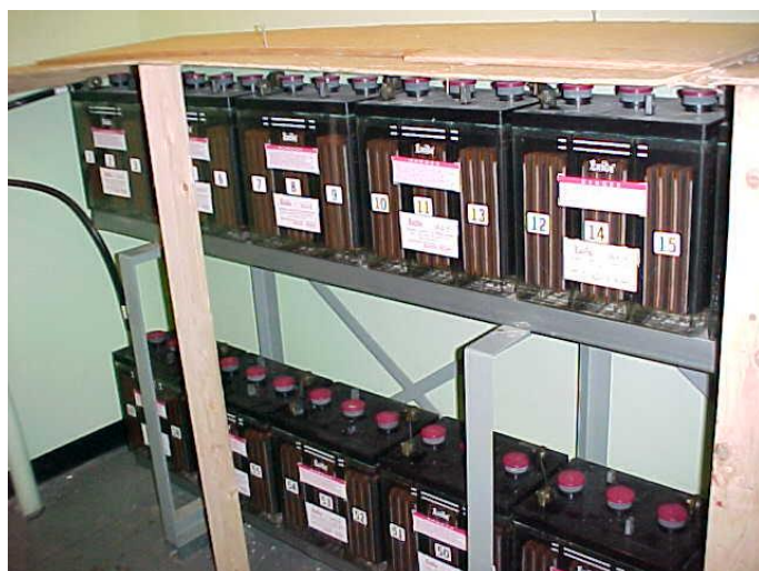
Figure 11: 125 V Direct Current Terminal Station Battery Bank
