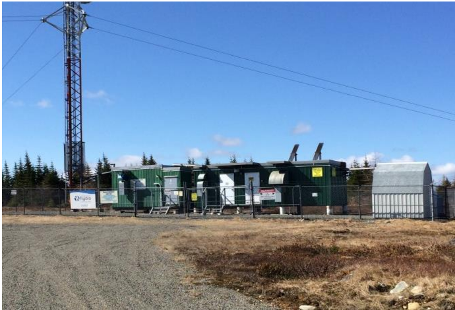
Figure 2: Gull Pond Hill Telecommunications Site
