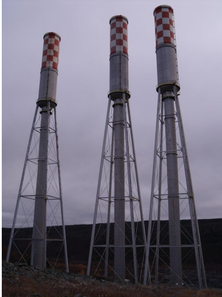
Figure 6: Surge Tanks at the Bay d'Espoir Hydraulic Generating Station
