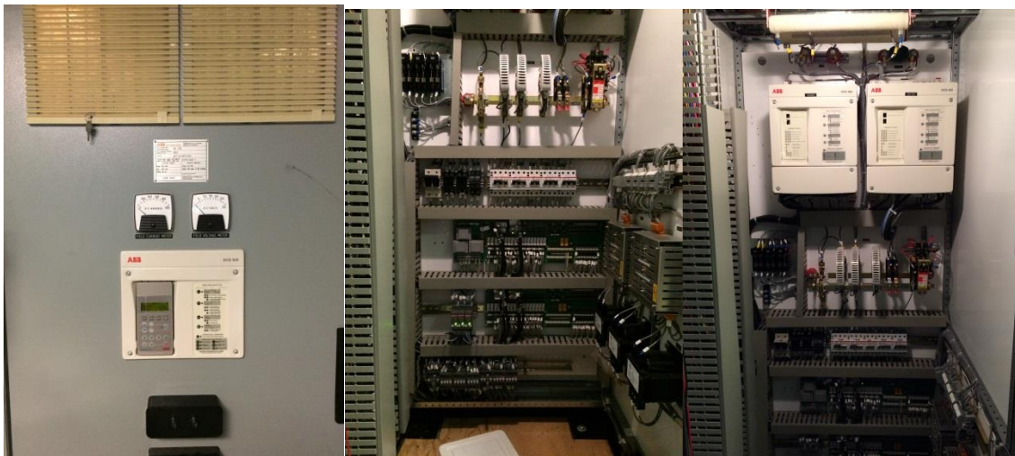
Figure 2: AVR Cabinet (Left to Right: Front, Inside Top, Inside Bottom)
