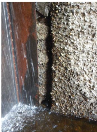
Figure 10: Concrete Deterioration - Ebbegunbaeg
