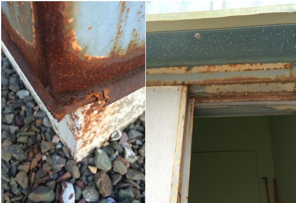
Figure 16: Building exterior cladding and doorways displaying severe rusting and deterioration
