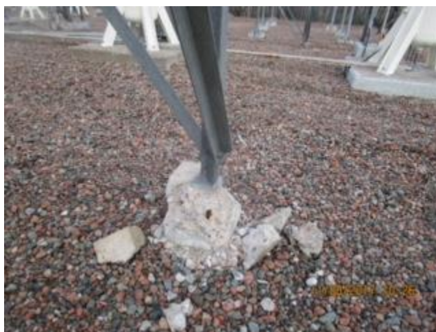
Figure 1: Compromised Foundation at Buchan's Terminal Station
