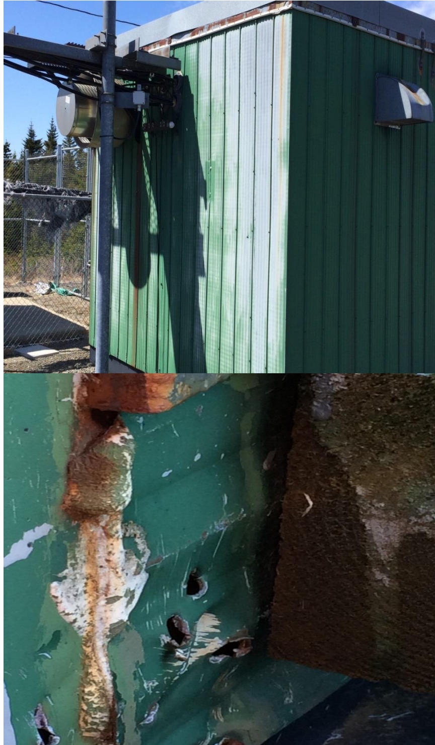
Figure 8A and 8B: Bay d’Espoir Hill – Deteriorated siding and rusted metal roof
