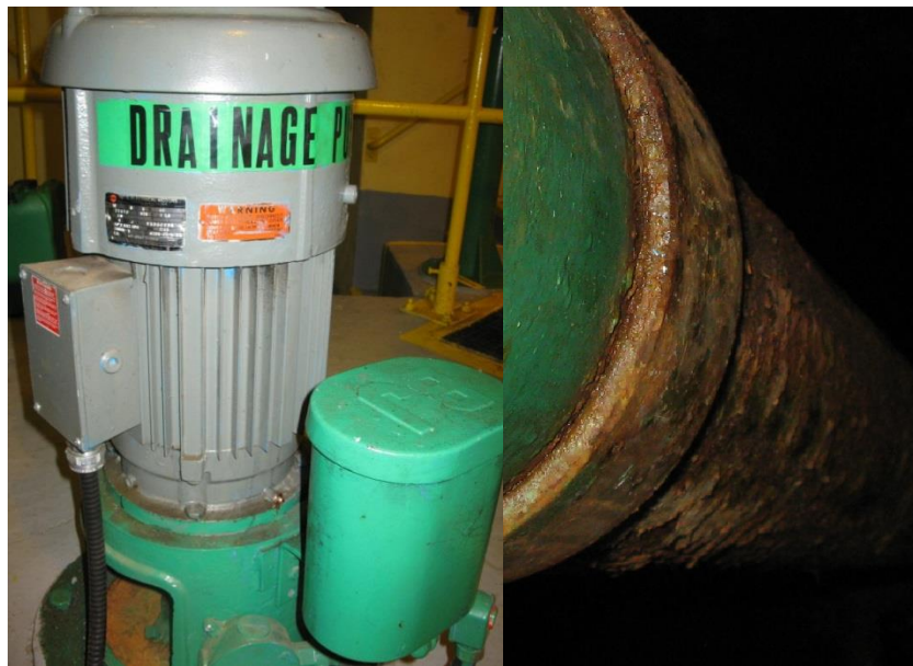
Figure 19: The drainage pump, motor, and column at Hinds Lake
