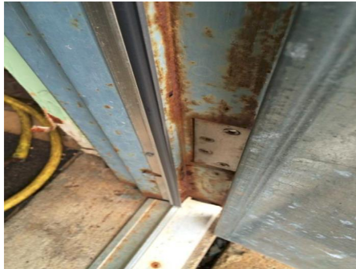
Figure 3: Rusted Doors at Holyrood
