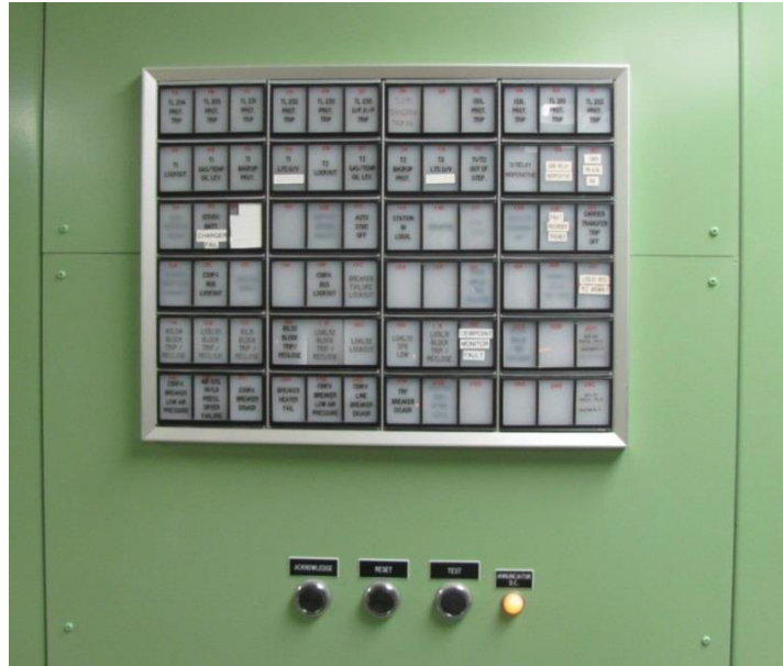
Figure 18: An annunciator commonly found in Hydro’s terminal stations
