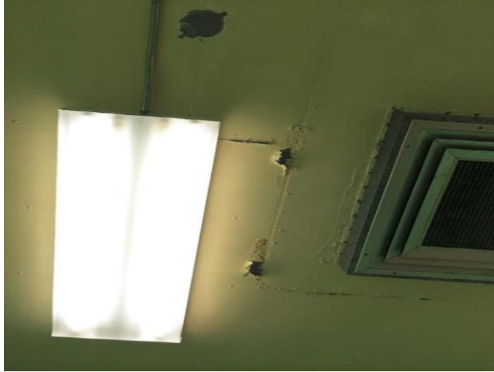
Figure 2: Leaking Roof at Holyrood
