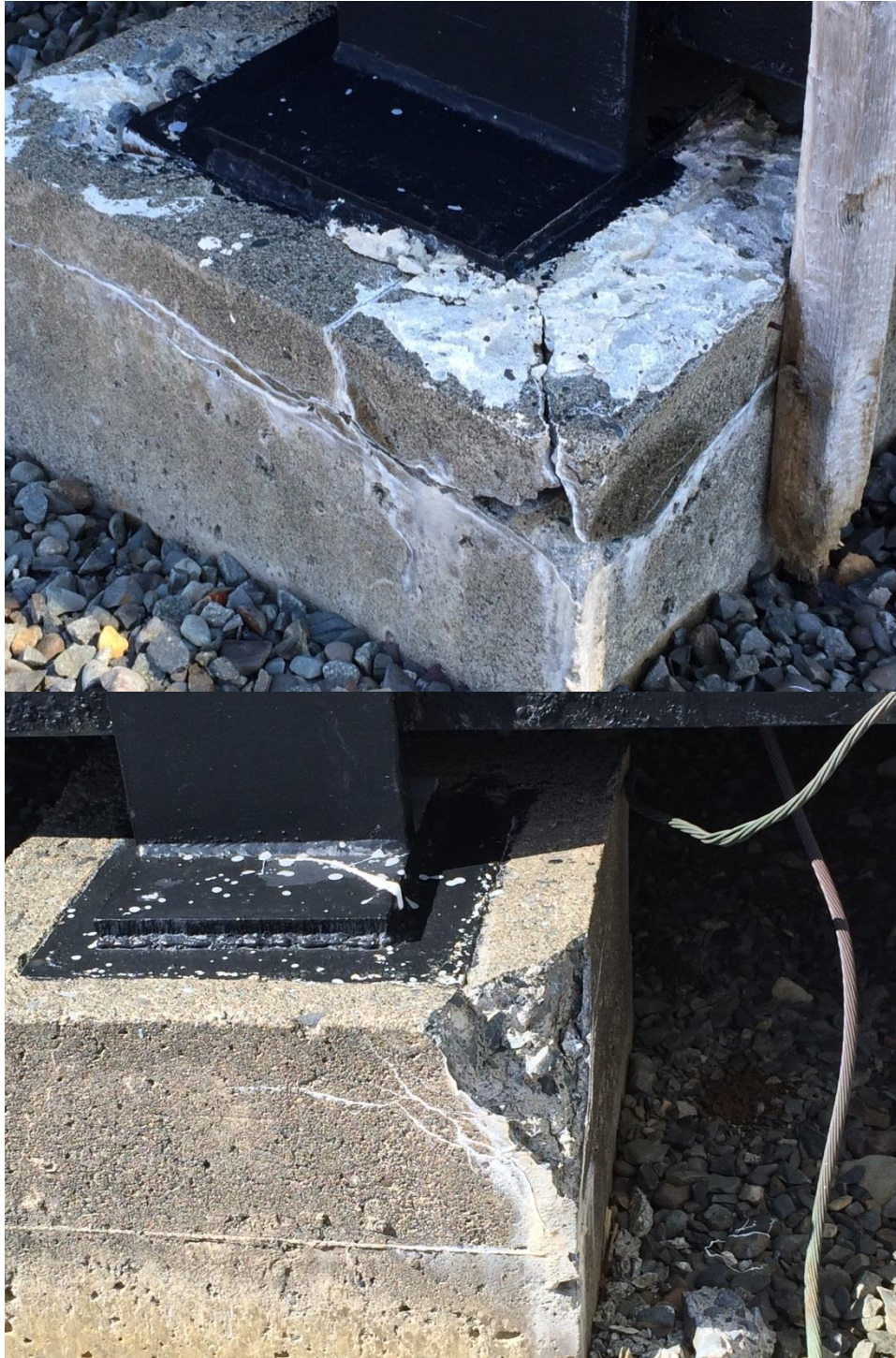
Figure 9A and 9B: Gull Pond Hill: Cracked and deteriorated building foundations
