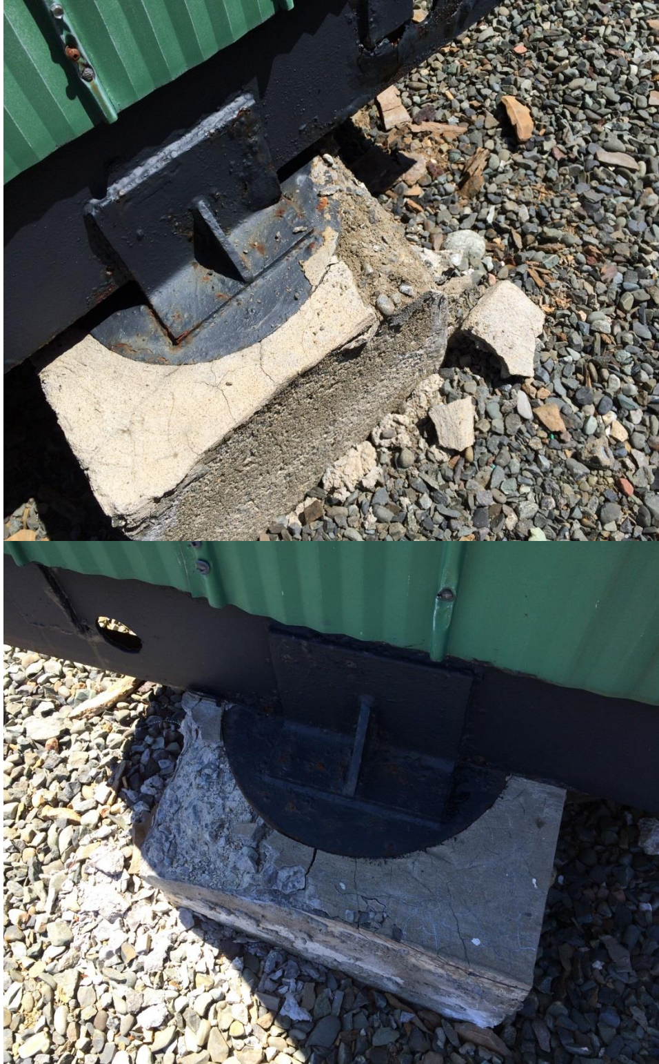
Figure 10A and 10B: Bay d’Espoir Hill – cracked and deteriorated building foundations
