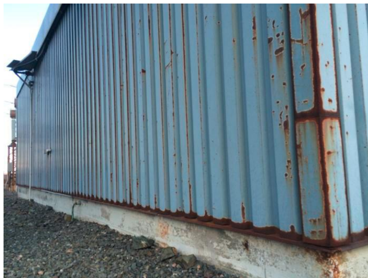
Figure 5: Rusting Exterior Cladding at Come By Chance
