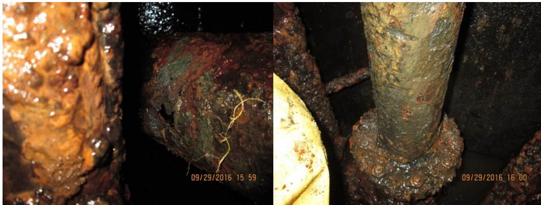
Figure 18: Corroded Component in the Paradise Sump
