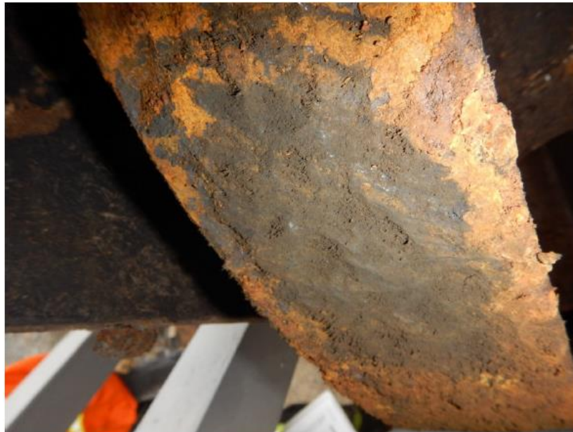
Figure 6: Pitting Corrosion on Main Rollers – Intake 1 2016
