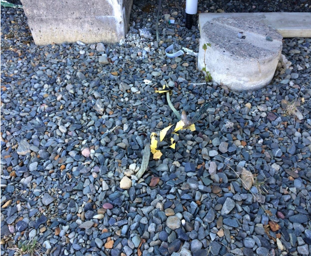
Figure 13: Gull Pond Hill – ground rod and wire above surface
