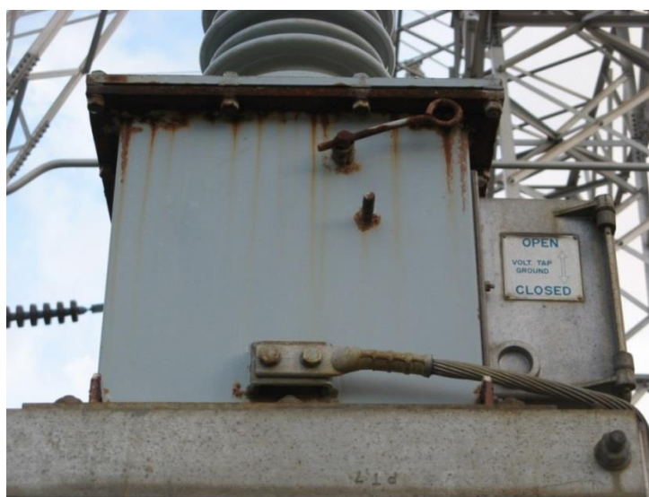
Figure 2: Rusting on Potential Transformer
