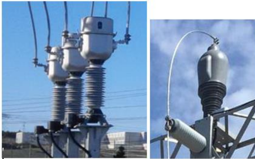
Figure 1: 69 kV Current Transformer (left) and Potential Transformer (Right)
