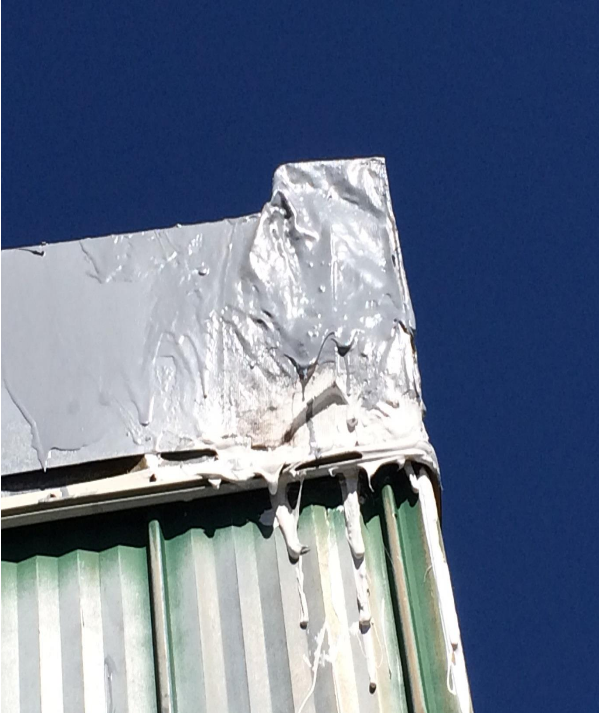
Figure 5: Gull Pond Hill – Temporary patching of metal roof to help prevent water entry
