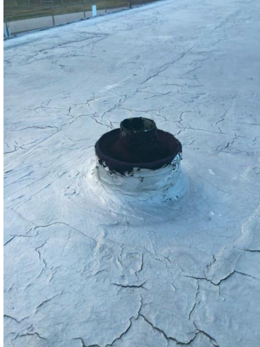
Figure 4: Roof Surface Cracking at Come By Chance
