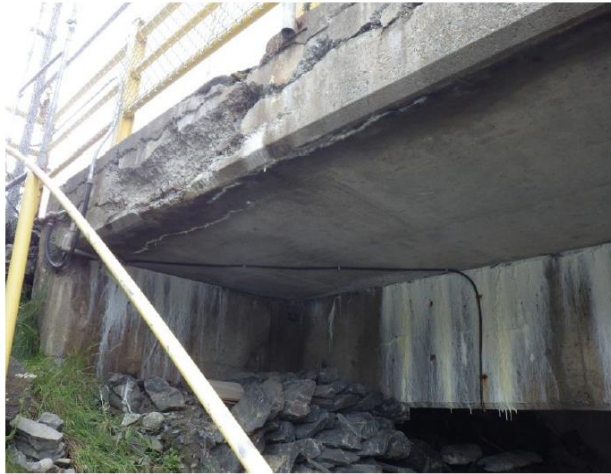
Figure 12: Deterioration on the Draft Tube Deck
